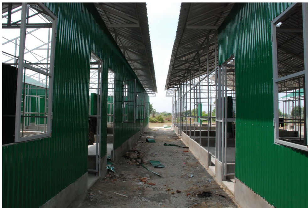
The housing at the resettlement site at Tuol Sambo is far from adequate: it is cramped and lacks basic amenities, including clean water supply.
