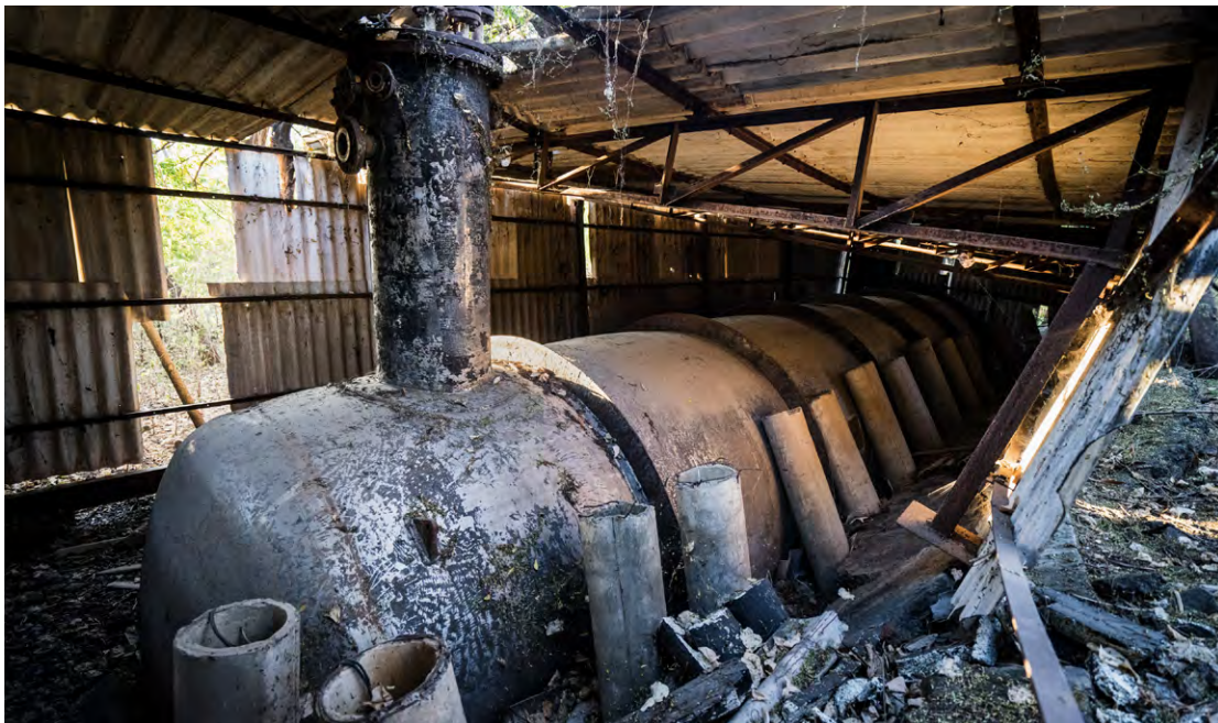
MIC holding tank at the derelict plant © Giles Clark 2014
