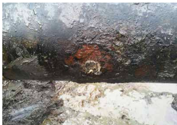
↑ Leak point on Eni's 8" Nimbe South-Obama flowline, 2014. Shell photograph.
