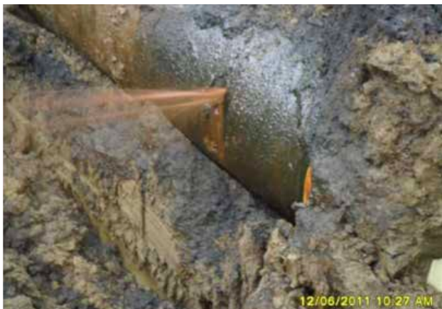
↑ Leak point on Shell's 24" Nkpoku - Bomu Pipeline at Biara, 2011 . Shell photograph.
